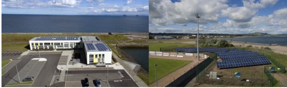
Figure 5-4: LCEP installed solar PV panels. 178 PV panels on roof of FIFE centre (left) and 440 PV panels on stadium ground. Courtesy of Bright Green Hydrogen
