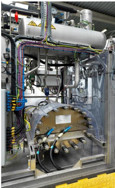
Figure 5-7: Hydrogenic PEM electrolyser installed in the LCEP. Courtesy of Bright Green Hydrogen
