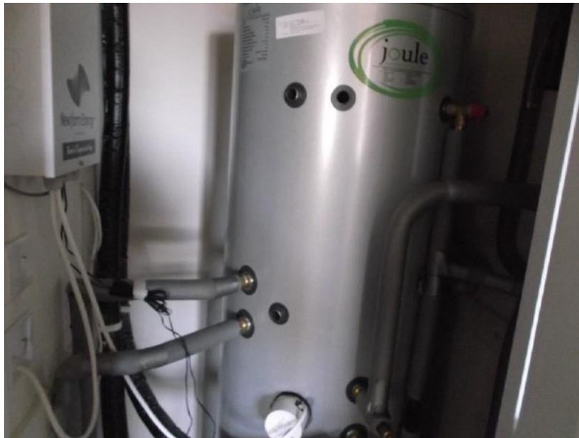
Figure 3-9: Modelled Hot Water Storage Tank. Courtesy of Electric Corby and EDP Consulting Limited[149].
