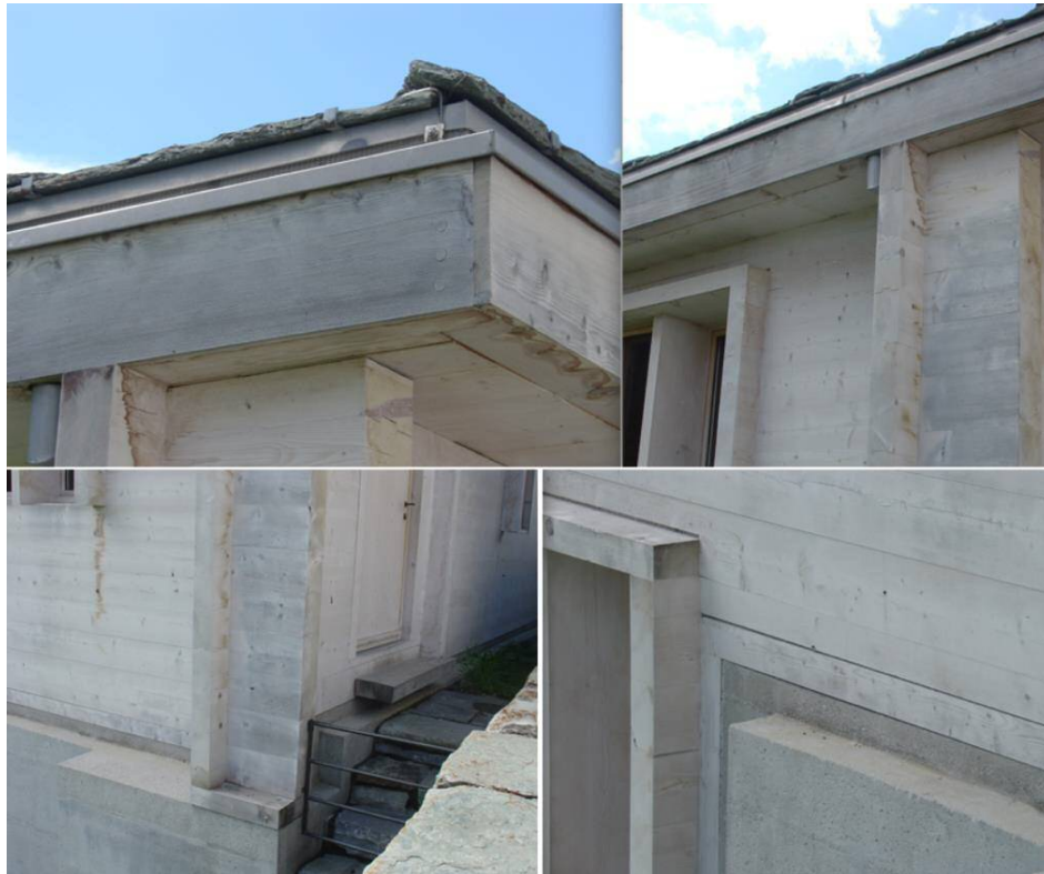
Figure 43: Detail designs. Upper: aluminium roof & slate tiles; lower: joint of timber and concrete
